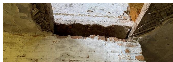
Figure 3 – First floor ceiling: 1 – finish floorboards, 4.5 cm thick; 2 – subfloor boards, 6.5 cm thick; 3 – joists, 30 cm wide, 22 cm high; 4–5 – lime plaster on lath
