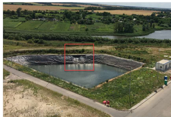
Figure 5 – Soil slope subsidence of south-west side of water basin
