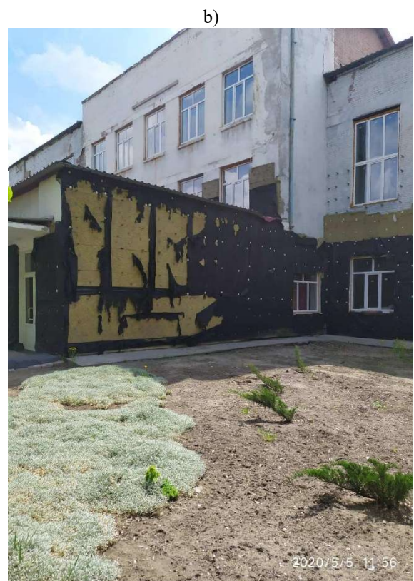
Figure 3 - Building in Rubizhne a – a fragment of the wall; b – a fragment of the facade with areas of complete destruction of mineral wool mats.
