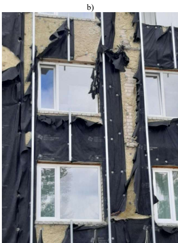
Figure 2 – Building in Starobelsk a – the state of unfinished construction; b – a fragment of the destroyed layer of mineral wool mats
