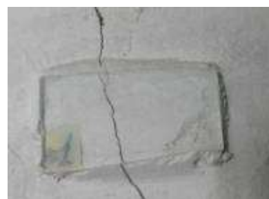
Figure 5 – Crack in the tell-tale (fifth floor)
