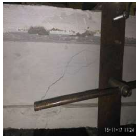
Figure 11 – General view of of an inclined crack at the edge
