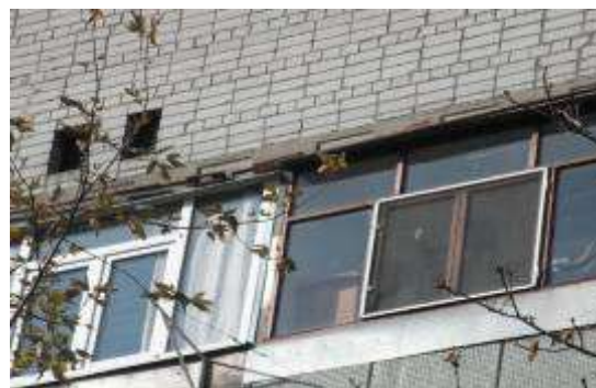
Figure 4 – Break of the upper tension bar along axis A at the level of the fifth floor overlap
