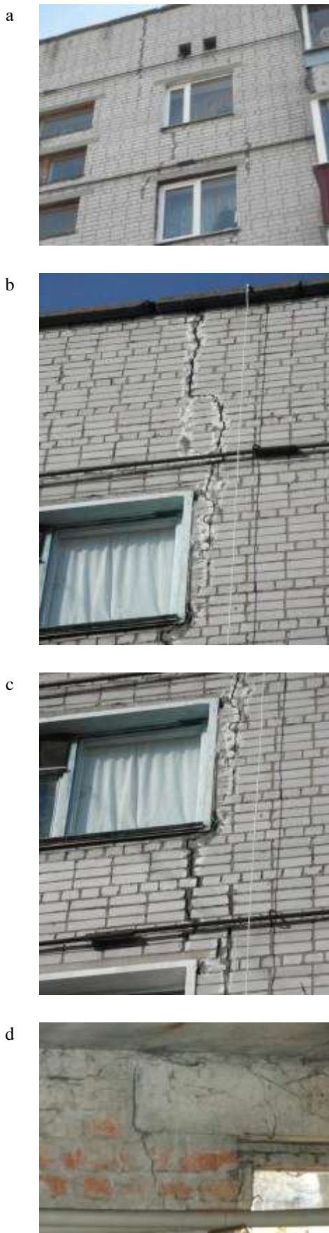
Figure 3 – Vertical cracks with opening width: a – 7 mm; b – 15 mm; c – 12 mm; d – 4 mm
