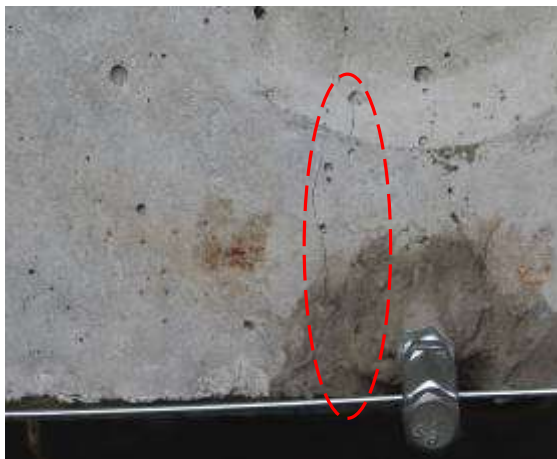
Figure 9 – Occurrence of the first cracks near the average cross section at a total load of 163 kN, such as pre-stressed PNC
