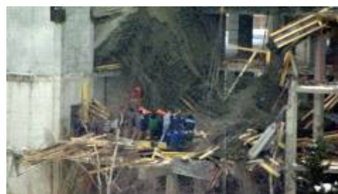
Figure 2 – Building collapse in Surgut, 2014
