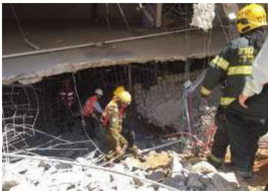
Figure 3 – Building collapse in Tel-Aviv, 2016
