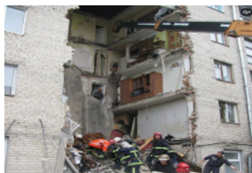
Figure 6 – Building collapse, Lutsk, Ukraine, 2012
