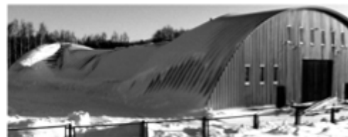
2014, The collapse of a warehouse (Russia)
