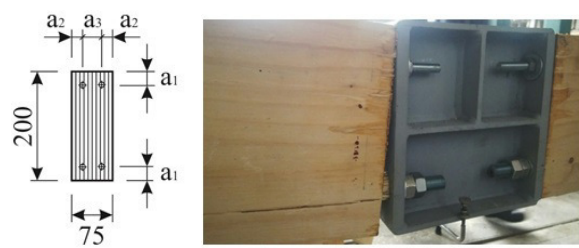
Figure 4 – The location of rods and the joint after destruction
