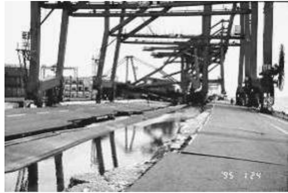
Figure 3 – Significant deformations of the berth territory from the earthquakes action
