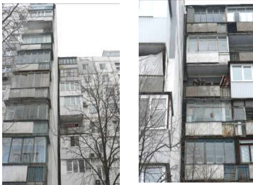
Figure 3 – The areas of house block-sections collision in a deformation joint
