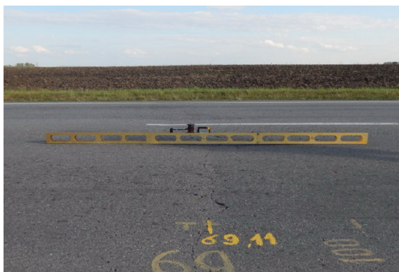
Figure 4 – Continuous transverse temperature crack at a characteristic section
