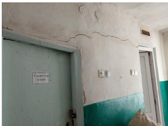
Figure 1 – Horizontal cracks on the walls
