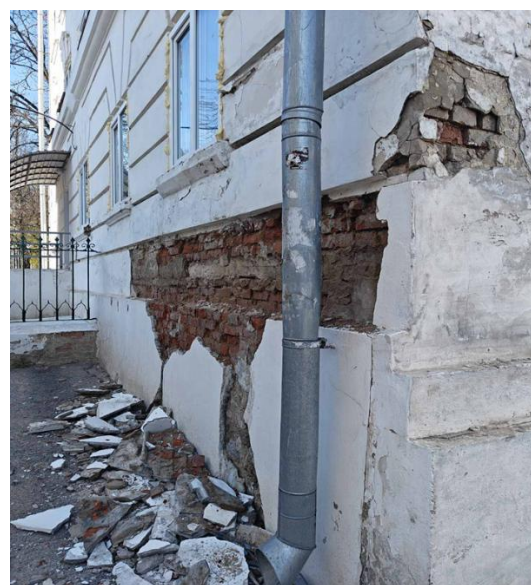
Figure 2 – Peeling of the plaster layer on the foundation and frost damage to the bricks
