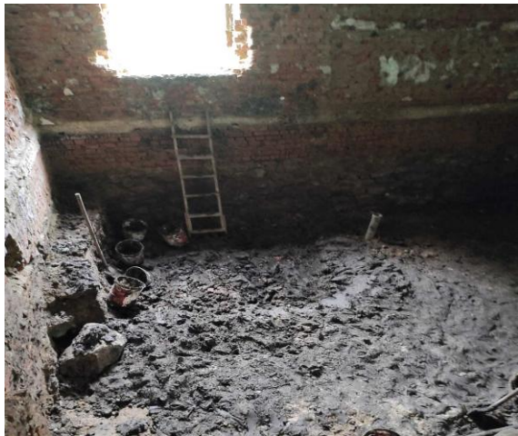
Figure 3 – Photographic documentation of water-saturated soil beneath the shower floor to a depth of 2.5 m from the 0.000 level
