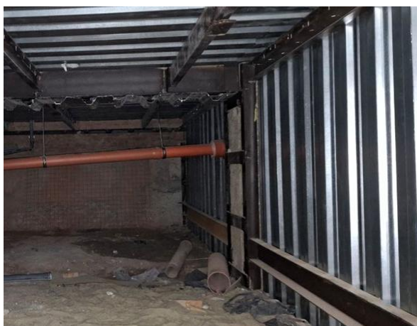
Figure 4 – General view of the basement with the interior brick wall reinforced by a layer of reinforced concrete using permanent formwork
