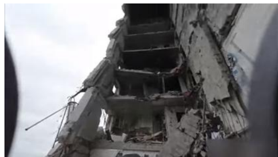
Figure 2 – Condition of a residential building in Severodonetsk
