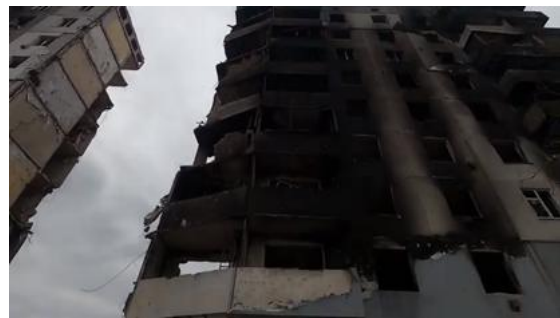
Figure 1 – Condition of a residential building in Borodyanka
