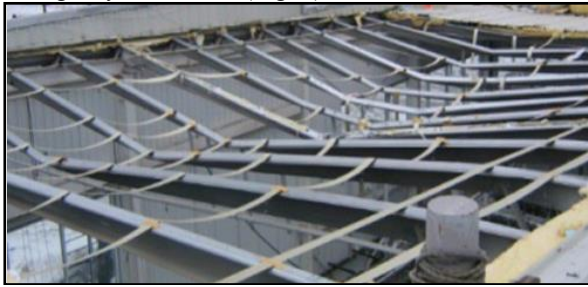
Figure 2 – Damage to roof from overloading
