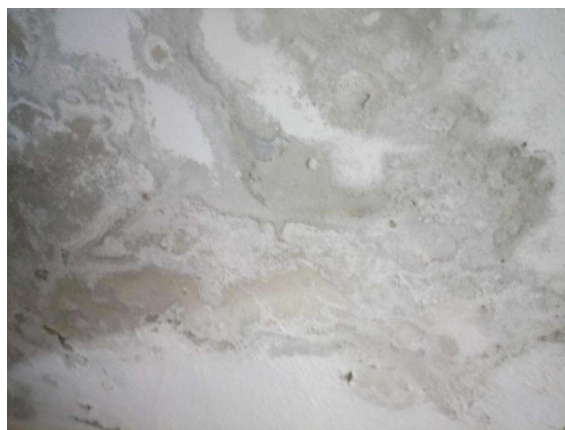
Figure 1 – Destruction of the plaster layer due to capillary moistening of foundations
