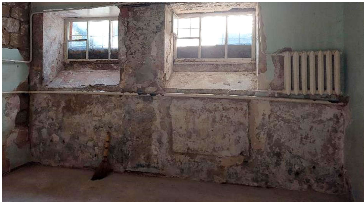
Figure 2 – Destruction of the inner surface of the walls of the basement room due to the rise of capillary moisture
