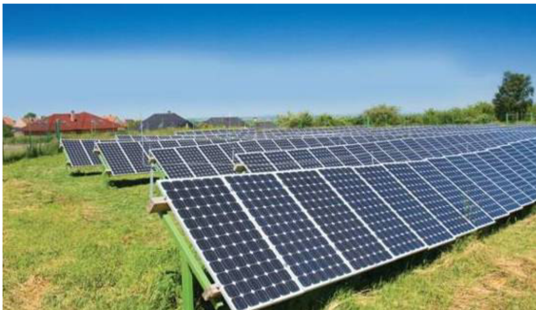
Figure 1 – Solar cell batteries at a private enterprise
